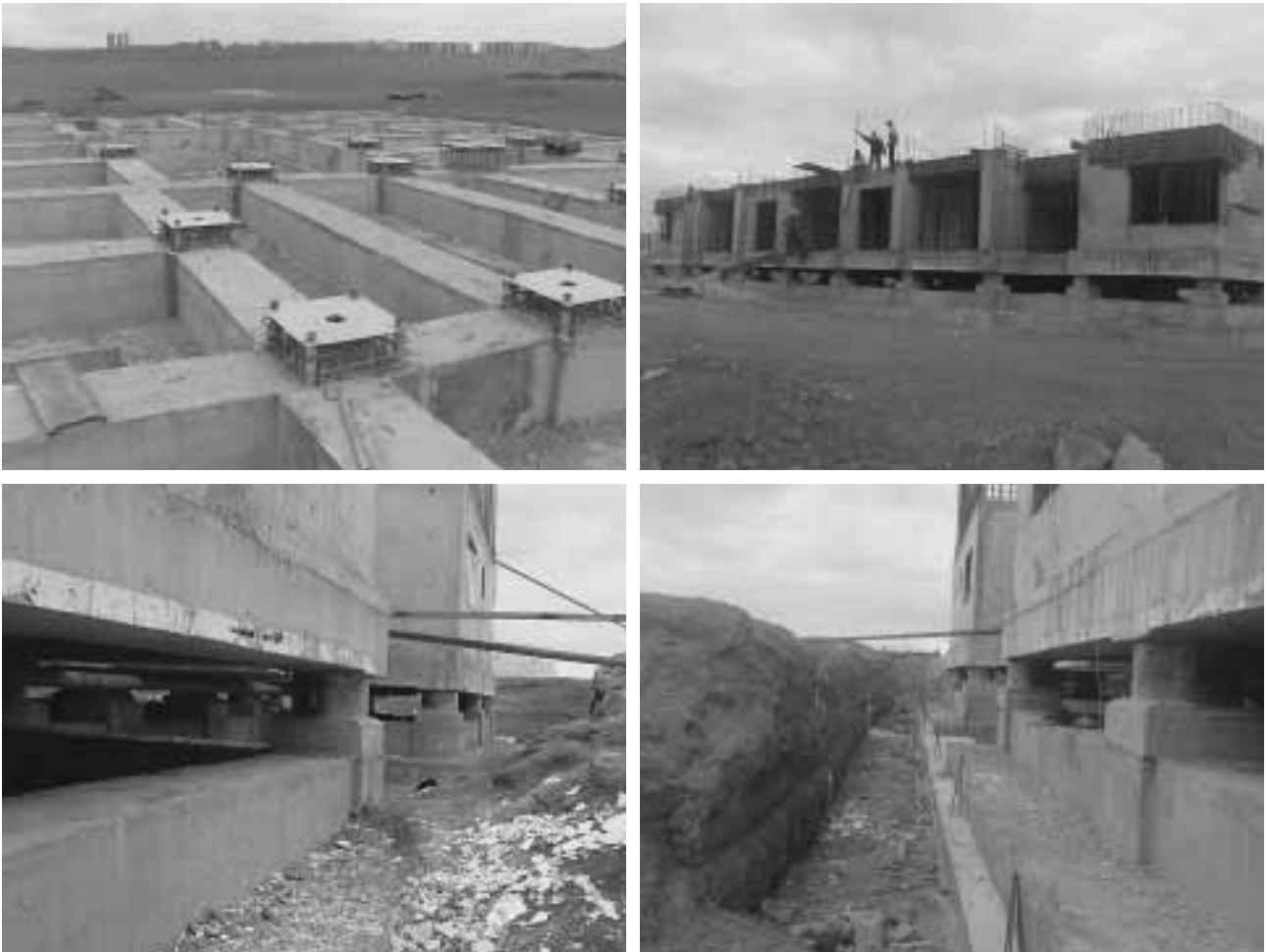
Figure 9. Typical 12 storey base isolated residential buildings under construction in Parand New Town near Tehran.
