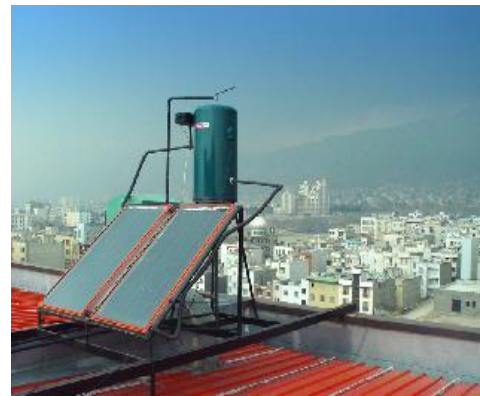
Fig. 6. A view of collector of water-heater type
