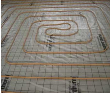
Fig. 8. A picture of heating pipes from the floor [5]
