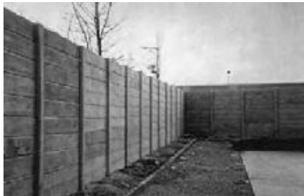
Figure 3. FRP reinforced post and panel fencing around a transmitter (courtesy EUROCRETE project).
