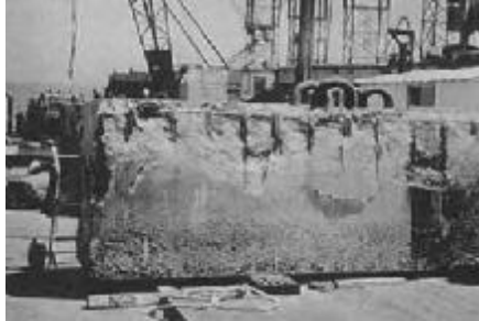
Figure 2. Damaged fender support beam, Qatar (courtesy EUROCRETE project).
